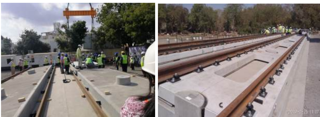
Laying of training Line with Slab Track at HSR Training Institute, Vadodara.
